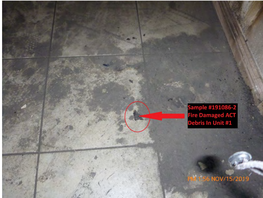
Photograph 7: November 15, 2019, at approximately 1:56 PM – Dry ACT debris on the floor of the north room of Unit #1. The material was sampled and later determined to contain 10% Chrysotile Asbestos.
