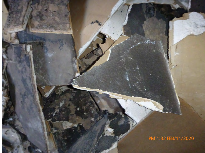
Photograph 11: February 11, 2020, at approximately 1:33 PM - View of textured drywall in a debris pile inside the north room of Unit 1. The material was sampled and later determined to contain 3% Chrysotile Asbestos by the point count method using polarized light microscopy. The material was in a dry condition with no evidence of moisture.
