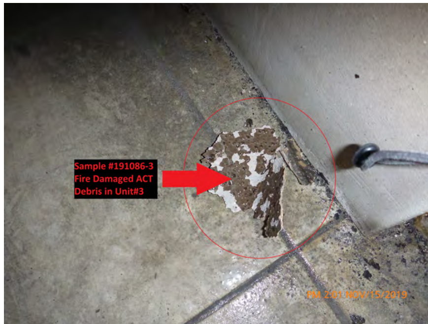
Photograph 14: November 15, 2019, at approximately 2:01 PM – View of ACT debris on the floor of the north room of Unit #3. The material was sampled and determined to contain 10% Chrysotile Asbestos.
