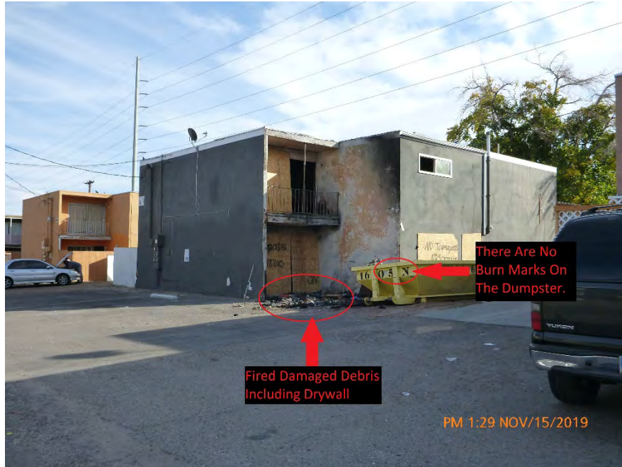
Photograph 1: November 15, 2019, at approximately 1:29 PM - View of the west side of 1480 E. Desert Inn Road, fire damaged debris on the ground, and a 16 cubic yard dumpster. The fire damaged debris included suspect asbestos-containing building materials. The dumpster was rented by Michael Perry who was also leasing the building.
