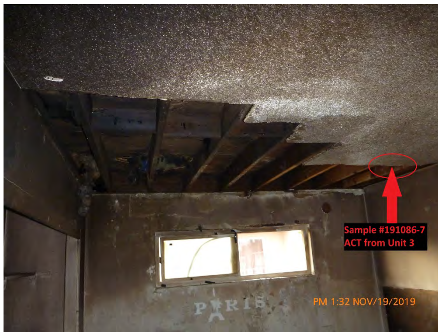
Photograph 18: November 19, 2019, at approximately 1:32 PM – View of ACT on the ceiling of the west room of Unit #3. The material was sampled and determined to contain 5% Chrysotile Asbestos.
