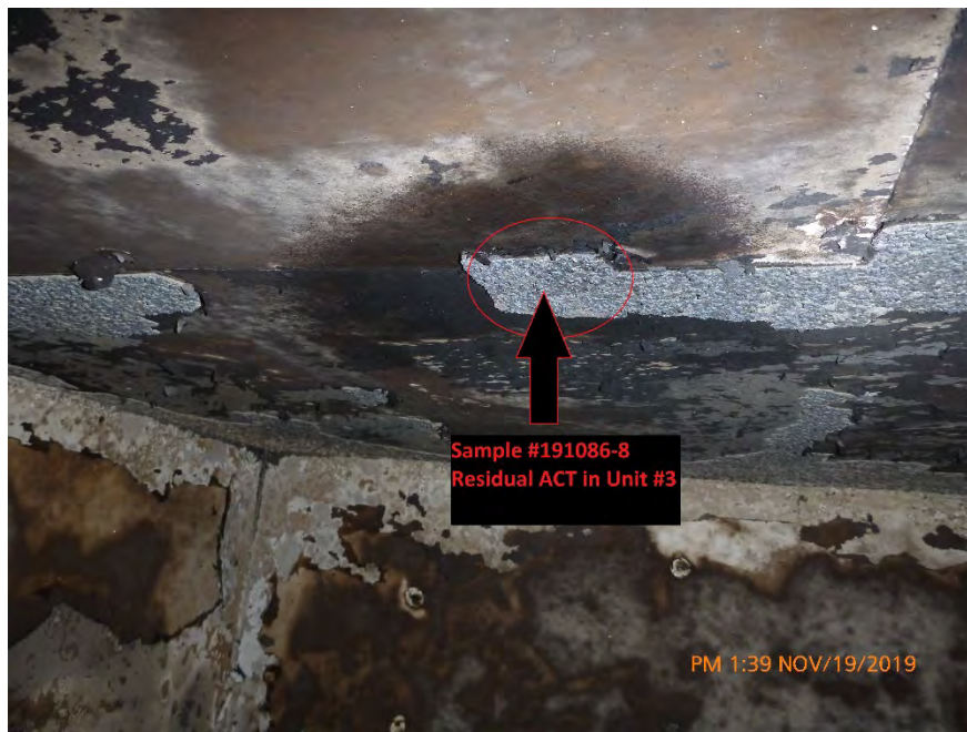
Photograph 16: November 19, 2019, at approximately 1:39 PM – View of Residual ACT on the ceiling of the north room of Unit #3. The material was sampled and determined to contain 5% Chrysotile Asbestos.
