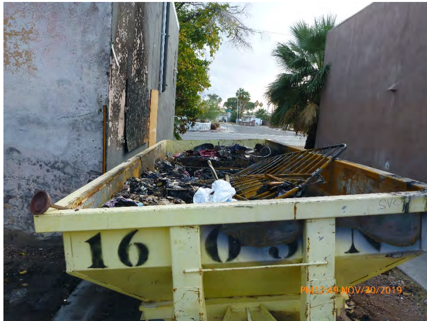
Photograph 23: November 20, 2019, at approximately 12:49 PM - View of the 16 cubic yard dumpster which contains ACWM. The dumpster remains uncovered and is not posted with asbestos warning signs.
