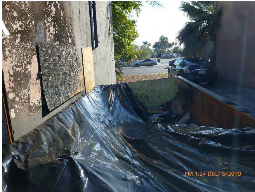
Photograph 28: December 5, 2019, at approximately 1:24 PM - View of the 16 cubic yard dumpster which contains ACWM. The dumpster is no longer sealed and debris has been removed (See Photograph #24 regarding the amount of material that was previously in the dumpster).
