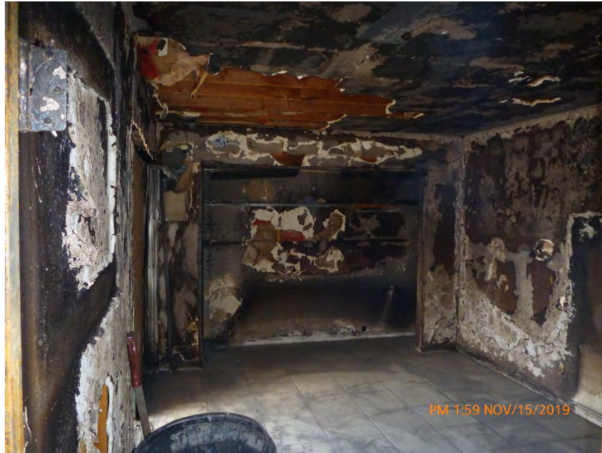
Photograph 11: November 15, 2019, at approximately 1:59 PM – View of the north room (master bedroom) of Unit #3. Nearly all of the ACT is missing and there are several holes in the ceiling. Despite the missing materials, the floor of the north room in Unit #3 contained almost no debris.
