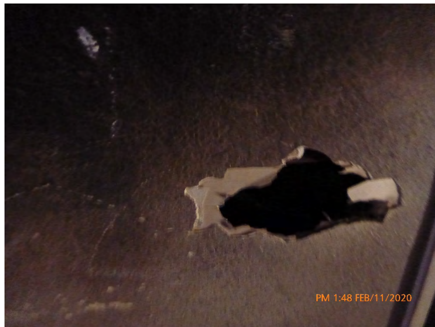
Photograph 15: February 11, 2020, at approximately 1:48 PM – View of textured drywall on the east wall of a hallway in Unit 1. The material was sampled and later determined to contain 2% Chrysotile Asbestos by the point count method using polarized light microscopy.
