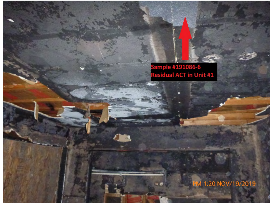
Photograph 9: November 19, 2019, at approximately 1:20 PM – View of the north room of Unit #1. Nearly all of the ACT is missing and there are several holes in the ceiling. Despite the missing materials, the floor of the north room in Unit #1 contained almost no debris (See Photograph #'s 6 & 7). The material was sampled and later determined to contain 5% Chrysotile Asbestos.
