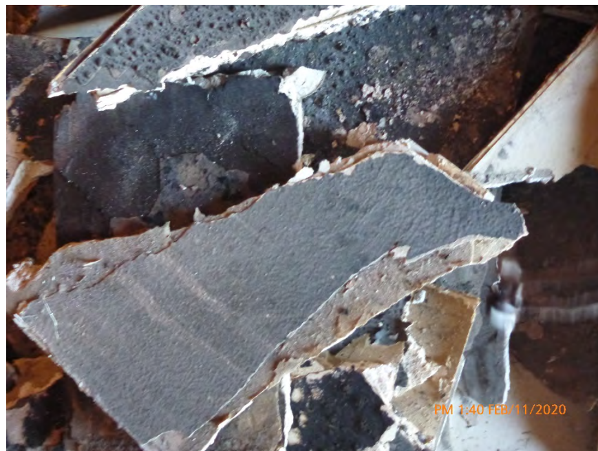
Photograph 13: February 11, 2020, at approximately 1:40 PM - View of textured drywall in a debris pile inside the north room of Unit 1. The material was sampled and later determined to contain 4% Chrysotile Asbestos by the point count method using polarized light microscopy. The material was in a dry condition with no evidence of moisture.
