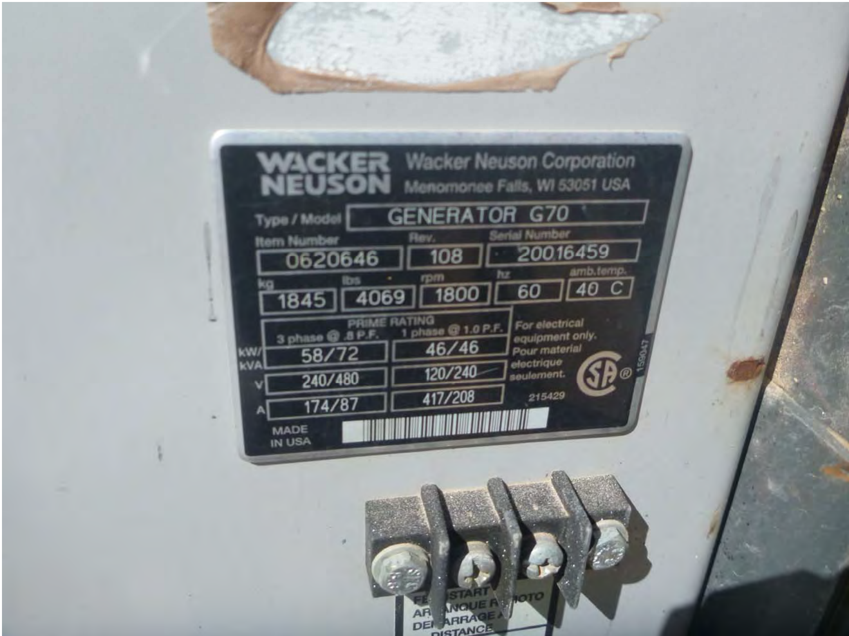
Photograph 7- Serial plate of Continuous Duty Diesel Engine (Generator) (EU: C06) depicting a 58 kW rating and Serial # 20016459. Photograph by Camon Liddell.
