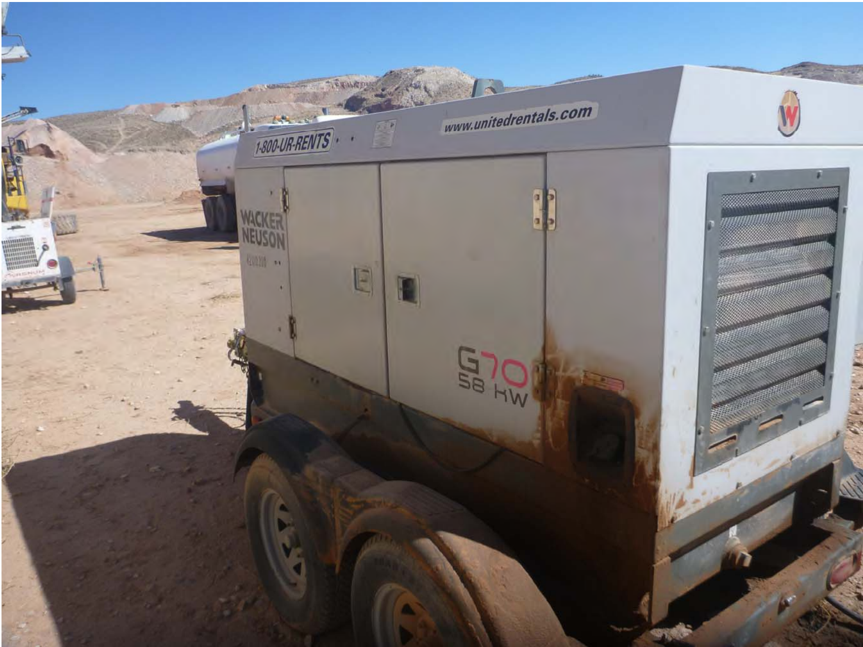
Photograph 6- Continuous Duty Diesel Engine (Generator) (EU: C06) [Maintenance]. Photograph by Camon Liddell.
