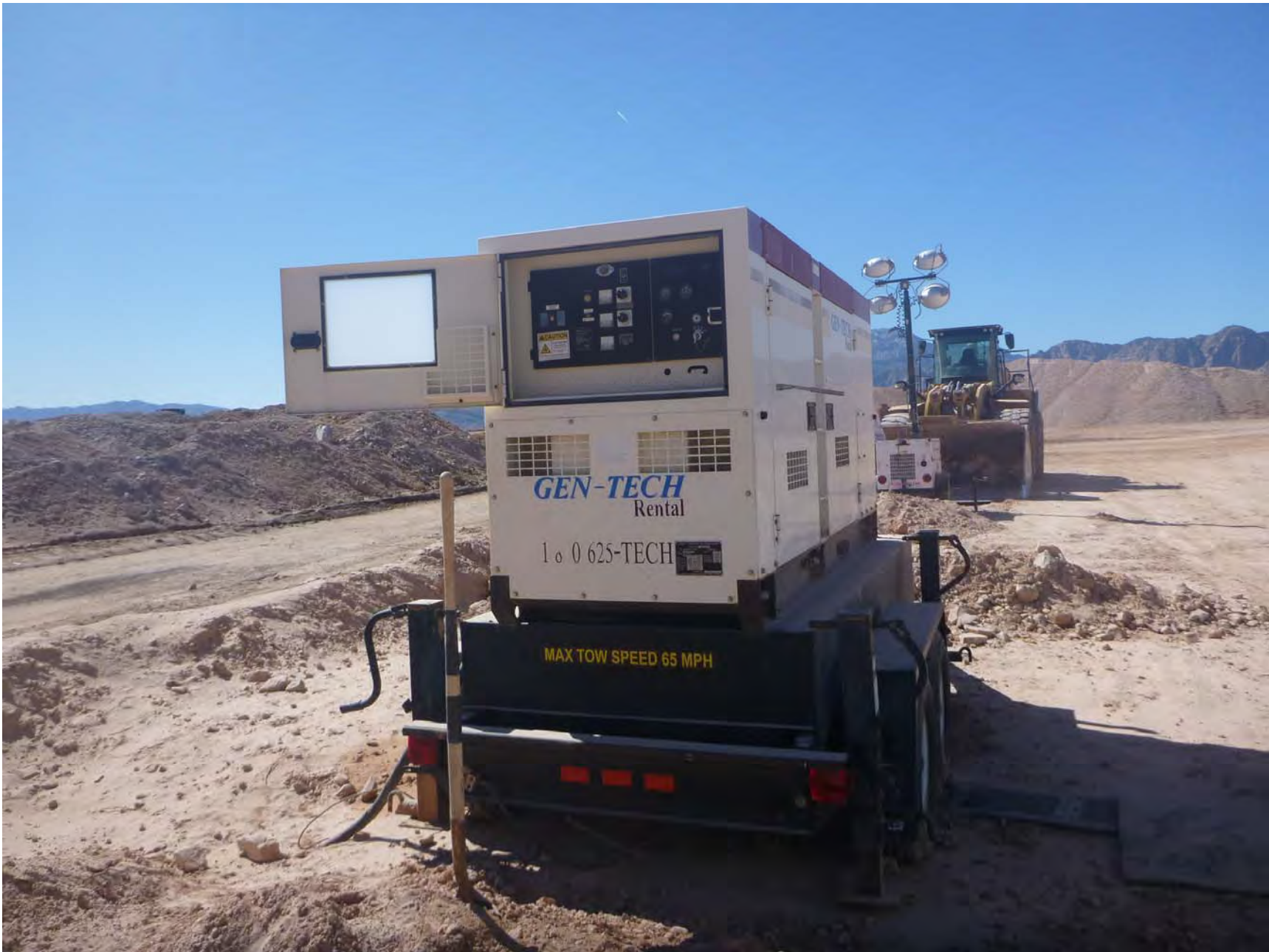
Photograph 9- Continuous Duty Diesel Engine (Generator) (EU: C05) [Loadout]. Photograph by Camon Liddell.
