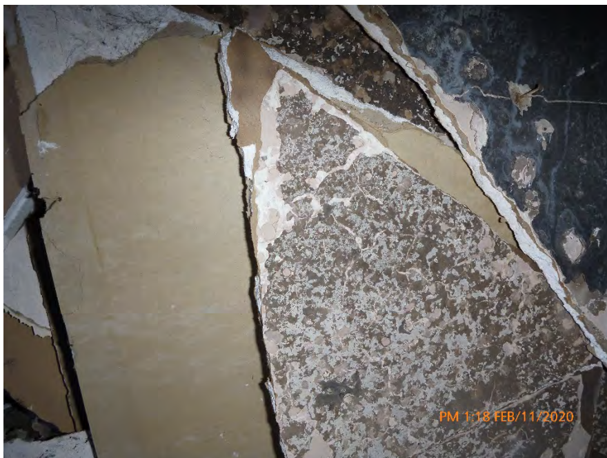
Photograph 5: February 11, 2020, at approximately 1:18 PM - View of textured drywall in a debris pile inside the north room of Unit 1. The material was sampled and later determined to contain 3% Chrysotile Asbestos by the point count method using polarized light microscopy. The material was in a dry condition with no evidence of moisture.
