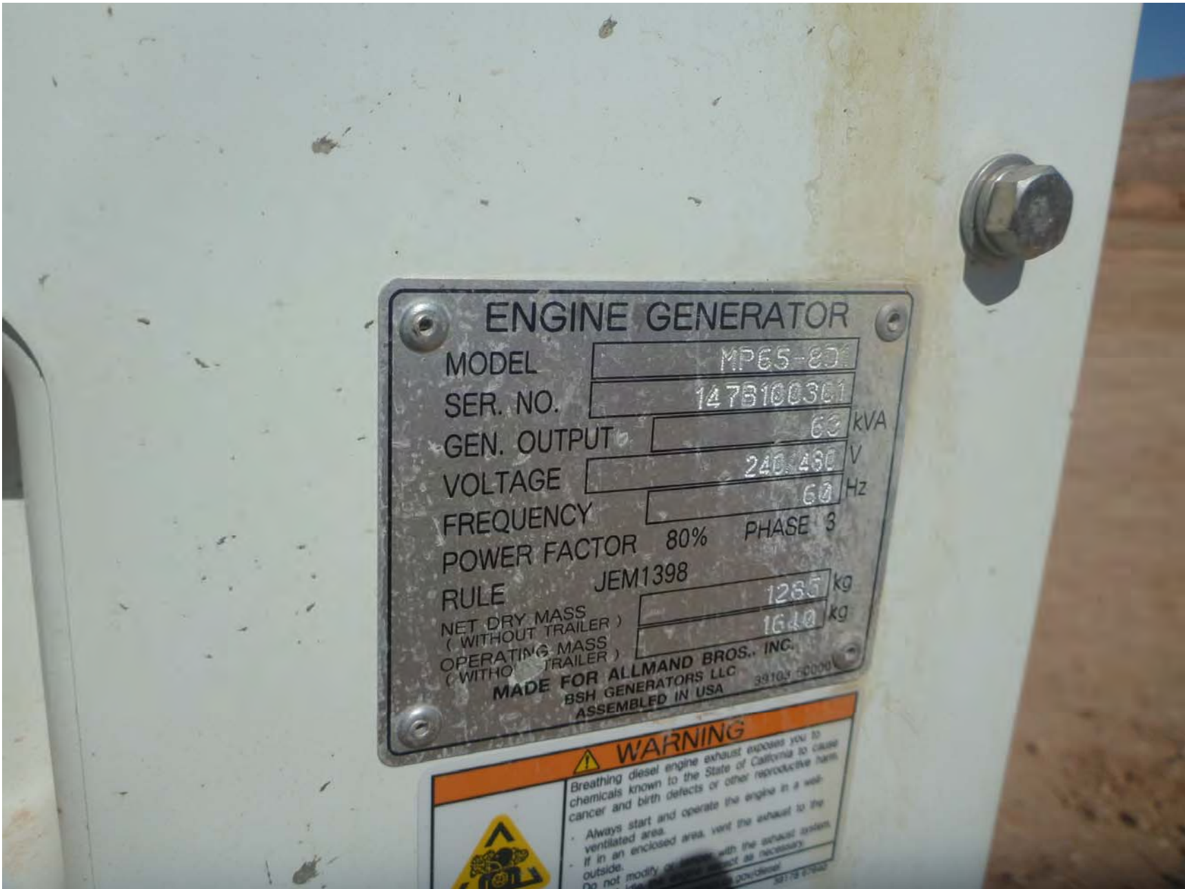
Photograph 12- Serial plate of Continuous Duty Diesel Engine (Generator) (EU: C08) depicting the Model # MP65-80. Photograph by Canon Liddell.
