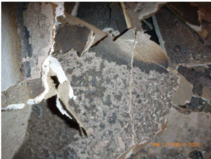
Photograph 7: February 11, 2020, at approximately 1:18 PM - View of textured drywall in a debris pile inside the north room of Unit 1. The material was sampled and later determined to contain 2% Chrysotile Asbestos by the point count method using polarized light microscopy. The material was in a dry condition with no evidence of moisture.
