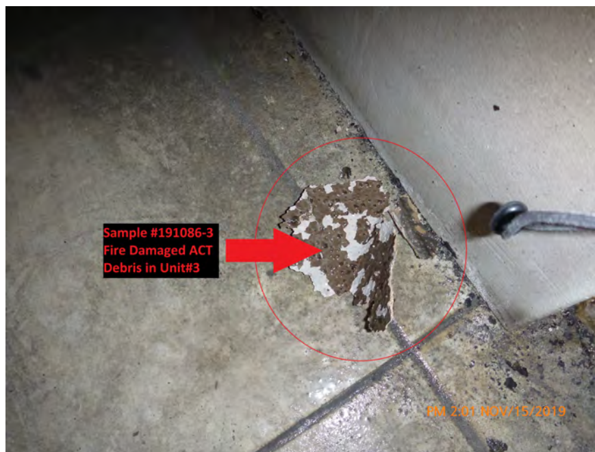
Photograph 14: November 15, 2019, at approximately 2:01 PM – View of ACT debris on the floor of the north room of Unit #3. The material was sampled and determined to contain 10% Chrysotile Asbestos.
