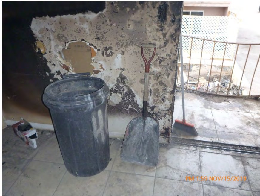
Photograph 12: November 15, 2019, at approximately 1:59 PM – View of a waste bin, a wide mouth shovel, and a broom in the north room of Unit #3. Note the absence of fire damaged debris in the photograph. Shovels like the one depicted in the photograph are typically used for the removal of materials such as soil, ash, ACT debris, etc...
