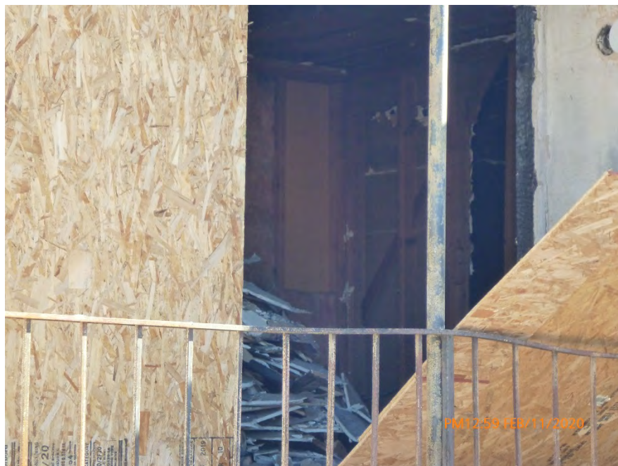
Photograph 3: February 11, 2020, at approximately 12:59 PM - View of the patio entrance to Unit 3. Plywood boards used to secure the entrance have been removed and no asbestos warning signs are posted. The Asbestos-Containing Waste Material inside is exposed to the outside air.
