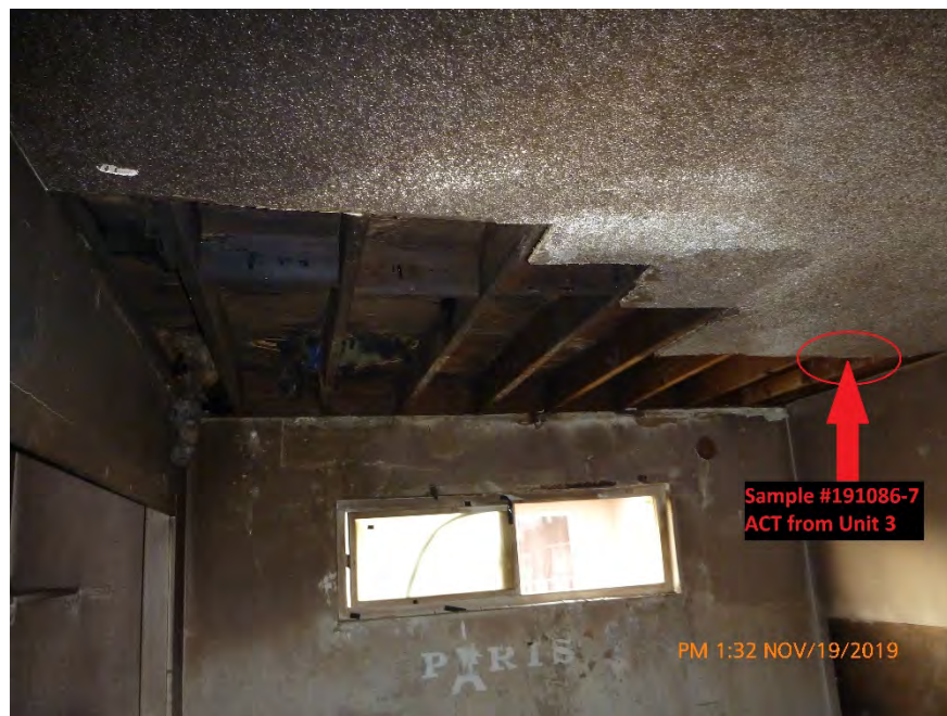
Photograph 18: November 19, 2019, at approximately 1:32 PM – View of ACT on the ceiling of the west room of Unit #3. The material was sampled and determined to contain 5% Chrysotile Asbestos.
